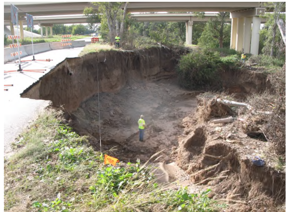
Fallwell Lane: $11.4M needed to stabilize bank
