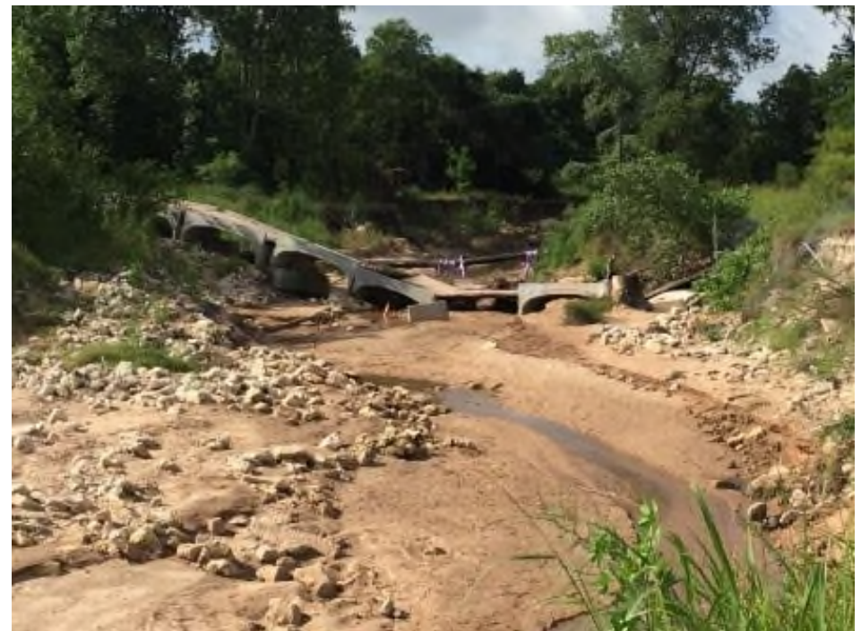
Roy Guerrero Park: Bridge destroyed
