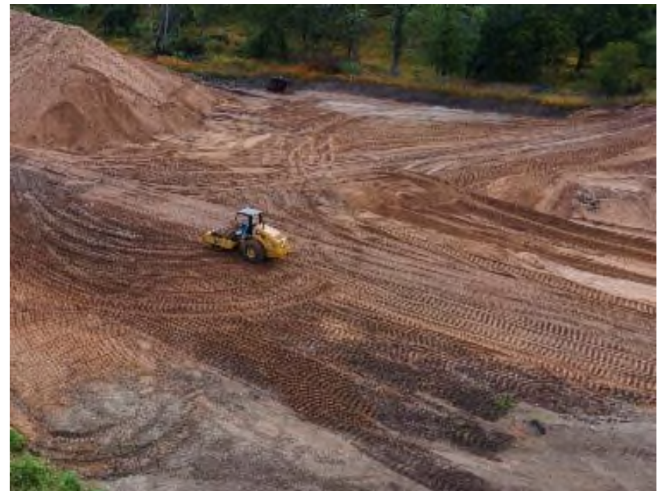
Roy Guerrero Park: $23M+ project to repair
