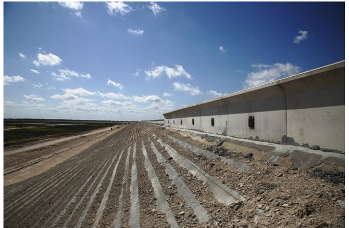
Custom-built concrete parapets along the top of the embankment will prevent wave action that could damage the reservoir.
