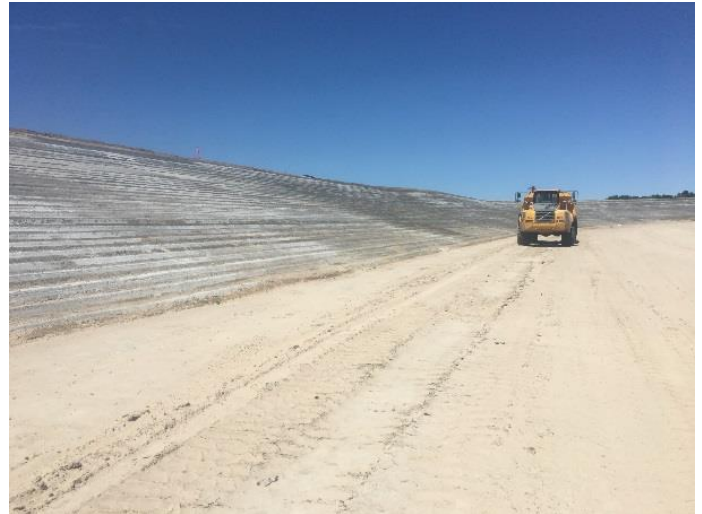
A truck waters down the sides of the new reservoir, which is strengthened with soil cement, during construction in 2017.
