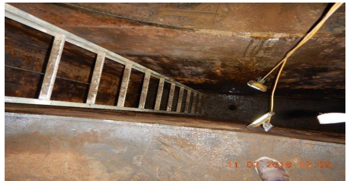
Crews must perform some of the rehab work in the small, narrow floodgate slots.
